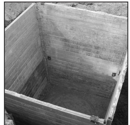
Two, 8x8x8 ft. stacked Modular Shields with Stacking Guides
